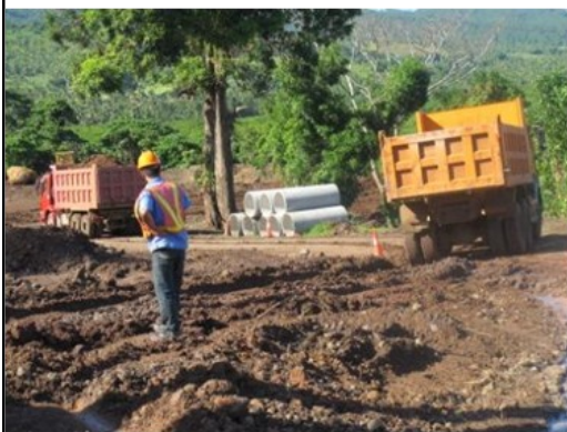
Left: Ongoing work on the Nabouwalu to Dreketi highway in Bua Province. Photo © Sirkka Killmann
